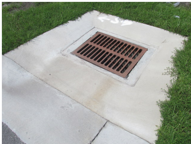
Catch basin and concrete collar
