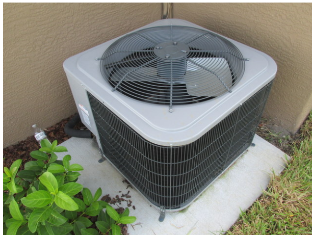
Split system condensing unit at clubhouse
