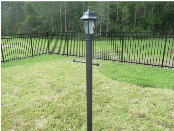
Light pole and fixture at pool area
