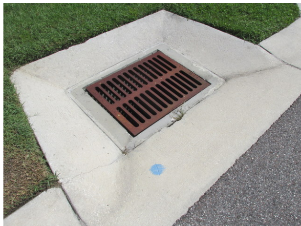
Catch basin and concrete collar
