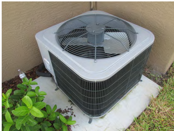
Split system condensing unit at clubhouse
