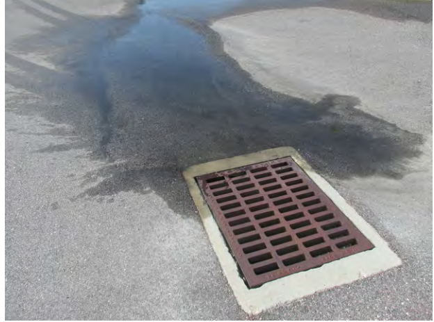
Inadequate drainage to catch basin at clubhouse parking area
