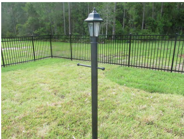
Light pole and fixture at pool area
